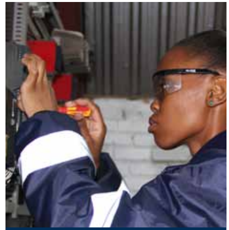
» Nelisiwe Vilakazi, Control & Instrumentation Apprentice pulling and wiring cables from the Programme Logistic Controller to the programme transmitter.
